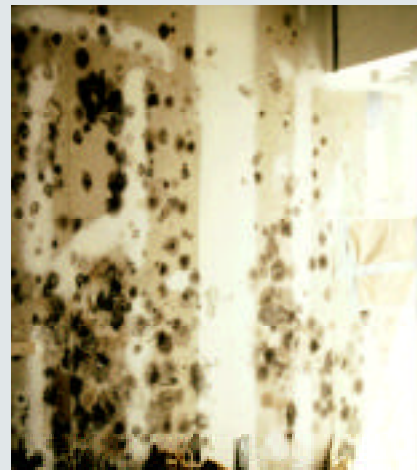
Mold growth on vinyl wall covering.
